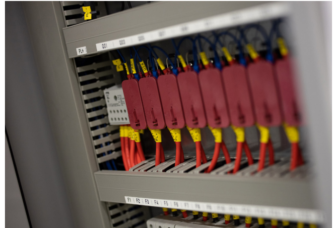
Close-up of contactors
